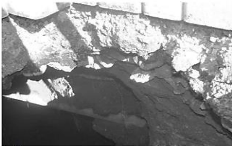
The entrance to the underground structures, formed near the store "Geese-Swans", Bar, 2012
